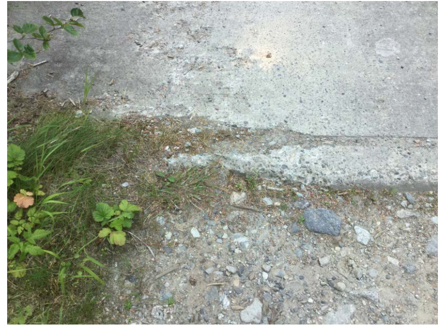
Ballast wall damage at right approach
